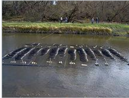
12-ton pond loop system being sunk to the bottom of a pond
