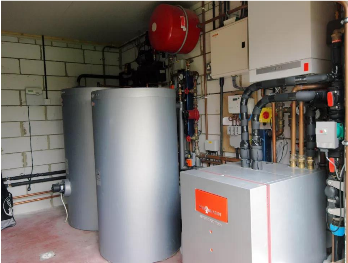
An example plant room in a home using a ground source heat pump from Viessmann
