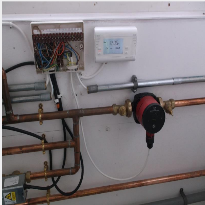
Task 3 Photo ref 7. Circulator installed, new cable and plug wired to the wiring centre and electrical supply restored.
