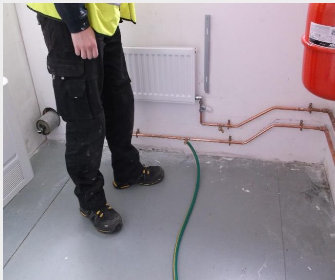
Task 2 Photo ref 17. Draining system with hose pipe to lowest drain in floor gully Hose was run across floor safely with Aboard signage
