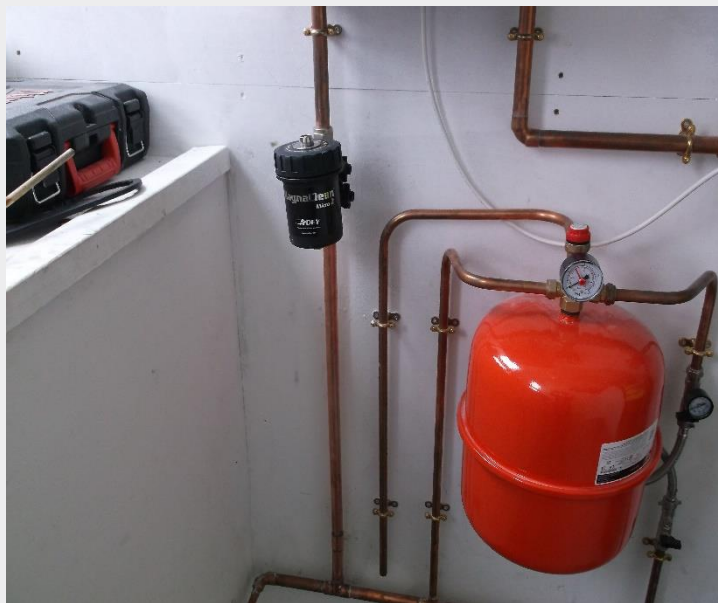
Task 2 Photo ref 2. Magnetic filter installed without any clips.
