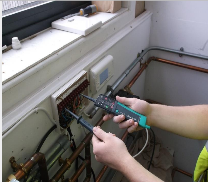
Task 3 Photo ref 2. Proving the Circulator line supply 230V
