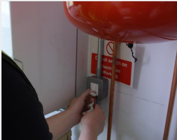
Task 3 Photo ref 3. Safe isolation of the heating system. Fuse removed and warning sign above switched fuse spur.
