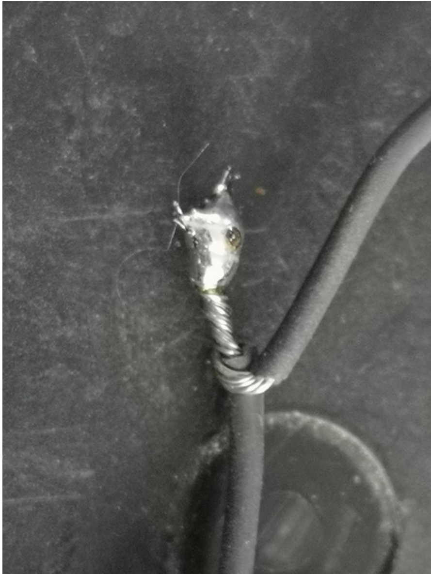
Photographs 4 and 5: Photographic evidence shows the wiring of the thermocouple head to the transmitter. Note, that the terminations show no nicks on the insulation, but the wire is stripped slightly too much leaving a small amount of exposed copper.
