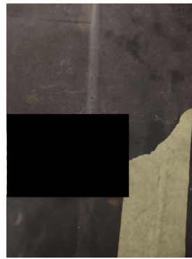
Taped backside of crack
