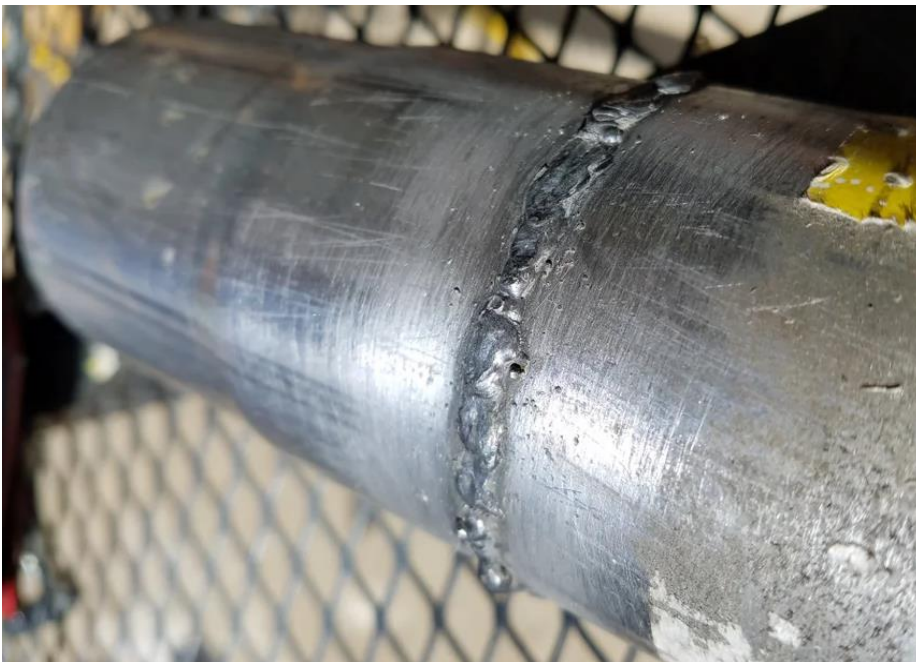
Photograph 2: Photographic evidence shows the welded joint between the exhaust pipe and extender, showing the level of quality finish with bubbles and a difference in weld thickness throughout the joint.
