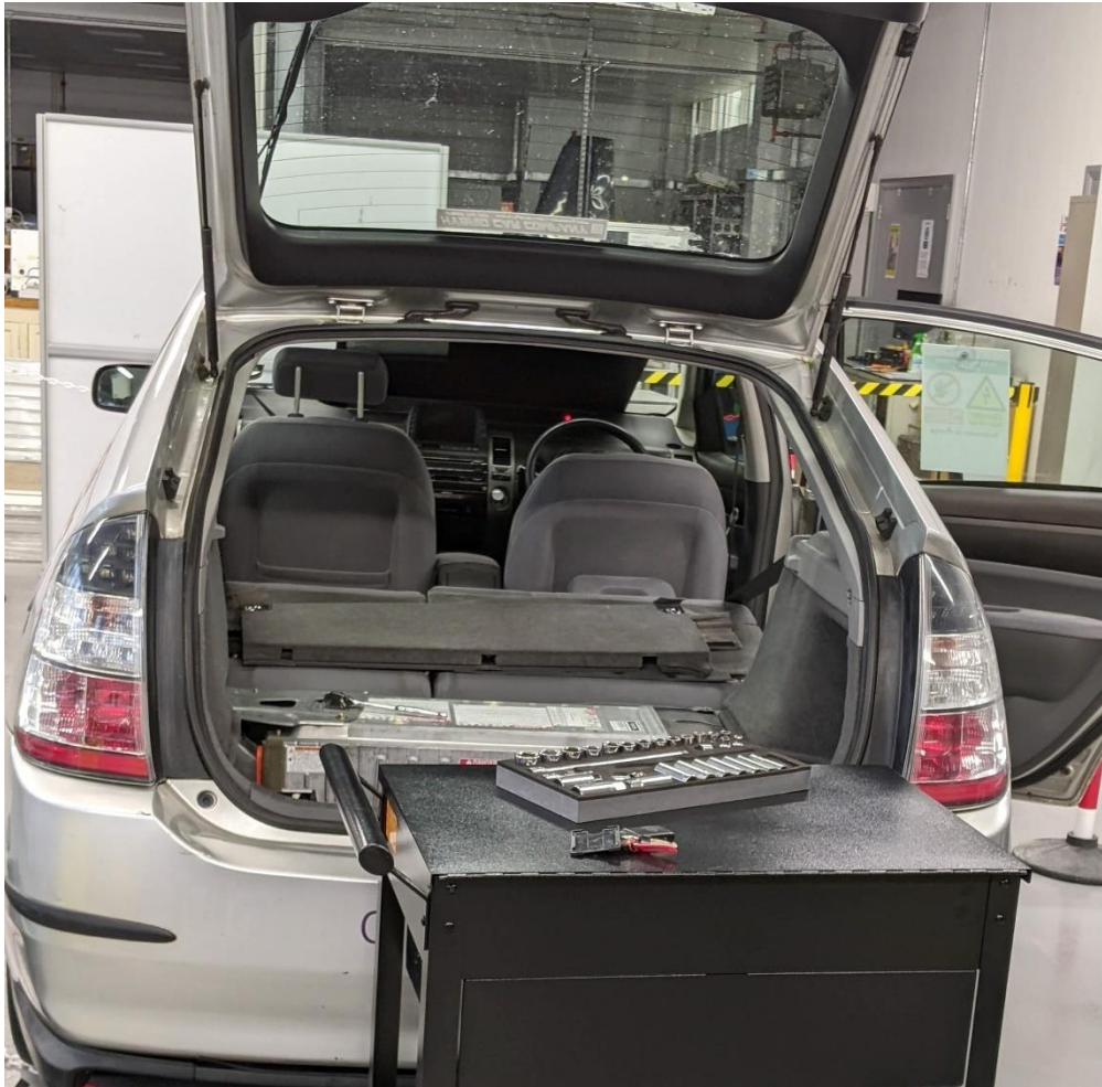
Photograph 3: Photographic evidence shows the high voltage battery correctly exposed with tools prepared but placed improperly.
