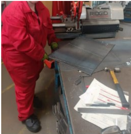
Marking out the metal to be able to cut the metal pieces
