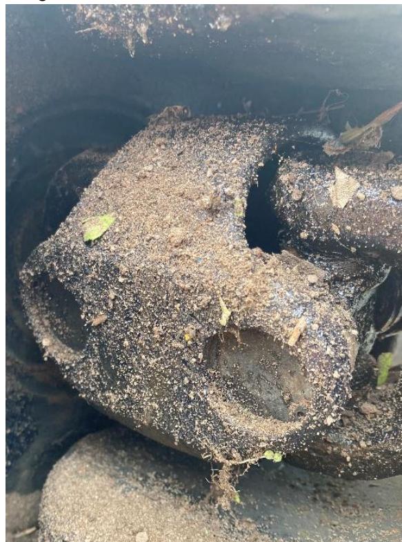
Photo 2 Condition of bearings and seals: before cleaned
