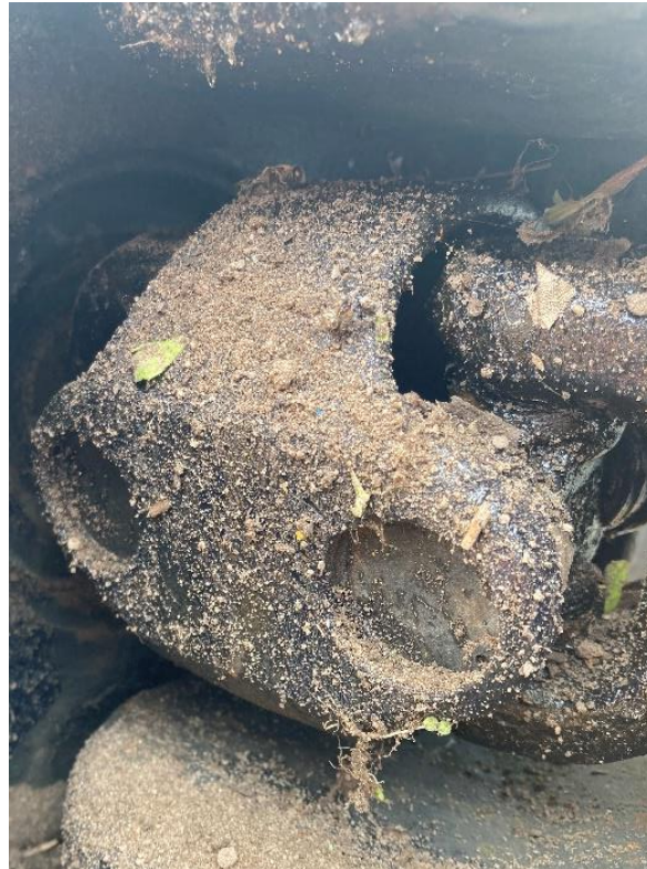
Photo 1 Condition of bearings and seals: before cleaned
